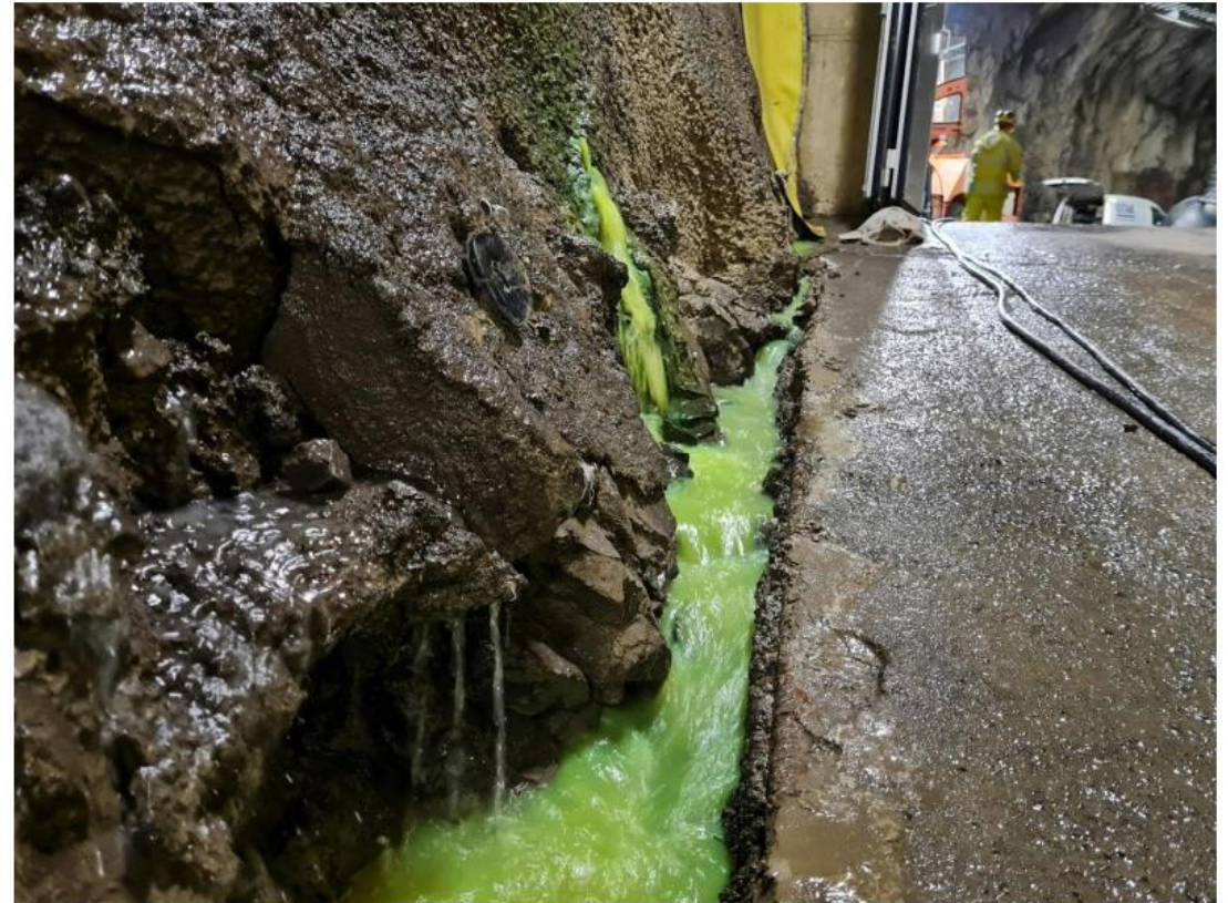
Figure 21. Leakage in right wall of the access tunnel to valve chamber with tracer pumped into joint at 10,5 m in BH06
